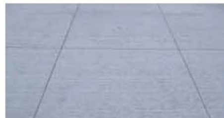
Concrete sidewalk Light broom finish, saw cut joints Tinted coloured concrete banding
