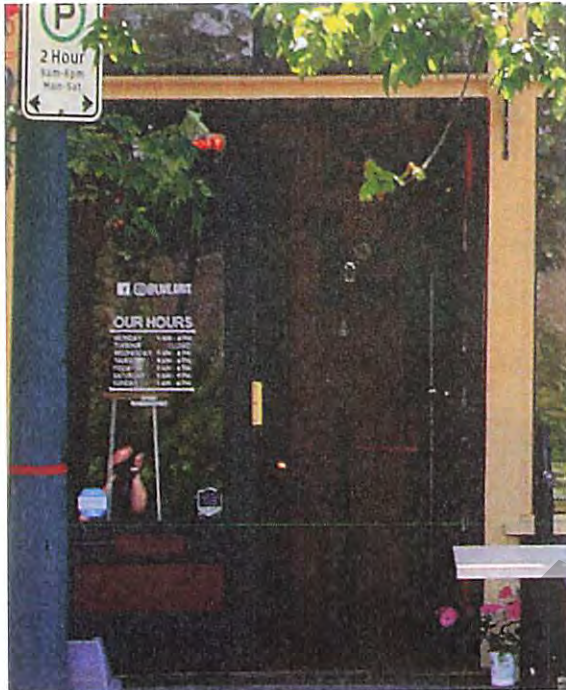
Existing double swing doors of main level commercial space facing Clarke Street. Note original metal mail slot on left paneled combination 3/4 glass and (1) One paneled door.
