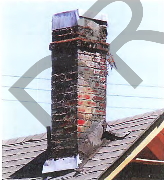
Extant chimney on the southwest side of the roof at the rear of the building.
