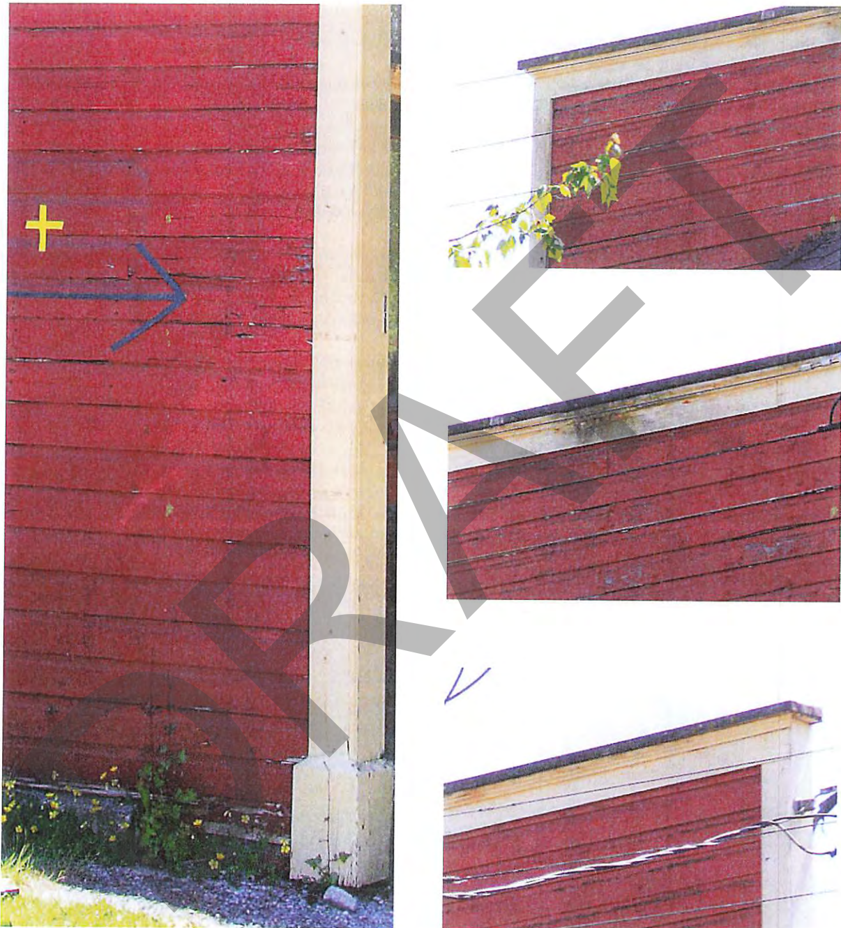
Current state of drop wood sidings on east and north elevations of the building. August 2021. Evidence of cracks, splitting, breaking of wood is visible. Peeling flaking and staining of paint on the facade after decades of exposure to the elements.
