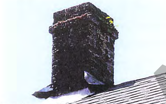
Extant chimney on the northeast side of the roof towards to front of the building at the apex of the gable roof
