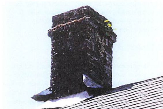
Extant chimney on the northeast side of the roof towards to front of the building at the apex of the gable roof
