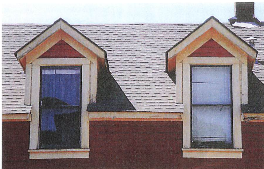
Two sets of extant roof dormers on the East and West elevations of the building with one-over-one, double-hung wood windows appear to have been restored and preserved. Further investigation to determine its condition to be done when possible.
