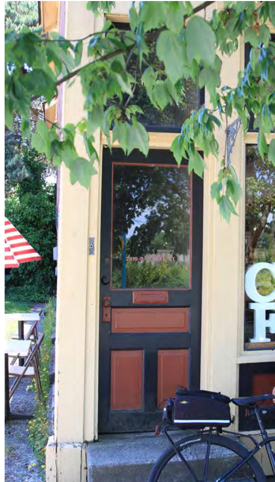
Original door opening on east side of the front elevation provides direct access from Clarke Street. Note metal mail slot, door hardware original to the paneled combination 2/3 glass and (3) Three panelled door.
