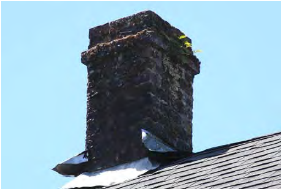
Extant chimney on the northeast side of the roof towards front of the building at the apex of the gable roof
