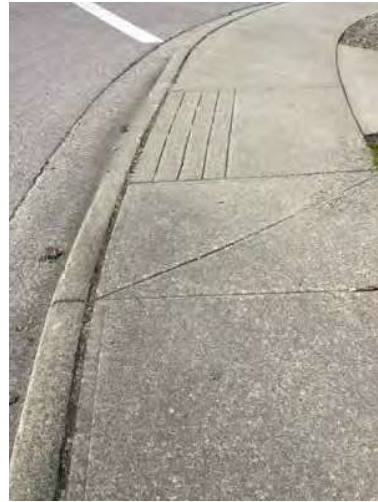
LOCATION 3 Example of curb cut slope very steep on northeast corner of St Johns Street at Moody Street. Accessibly challenged pedestrians have difficulty navigating, particularly with Moody Street a key route to Clarke Street.
