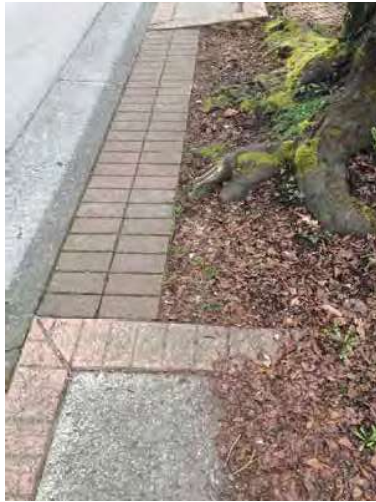
LOCATION 2 Example of curb condition on St Johns Street near Mary Street. Difficult for pedestrians to navigate, and harder still for those with accessibility concerns.
