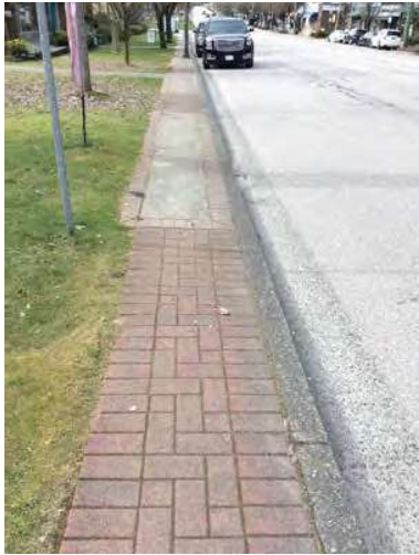
LOCATION 1 Pavement condition near curb on St Johns Street. Very narrow path and uneven paving bricks and landscaping. Extremely poor condition for pedestrians with accessibility issues.
