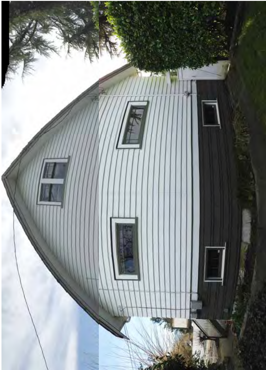
West elevation (two panorama images digitally merged due to site constraints), March 2016
