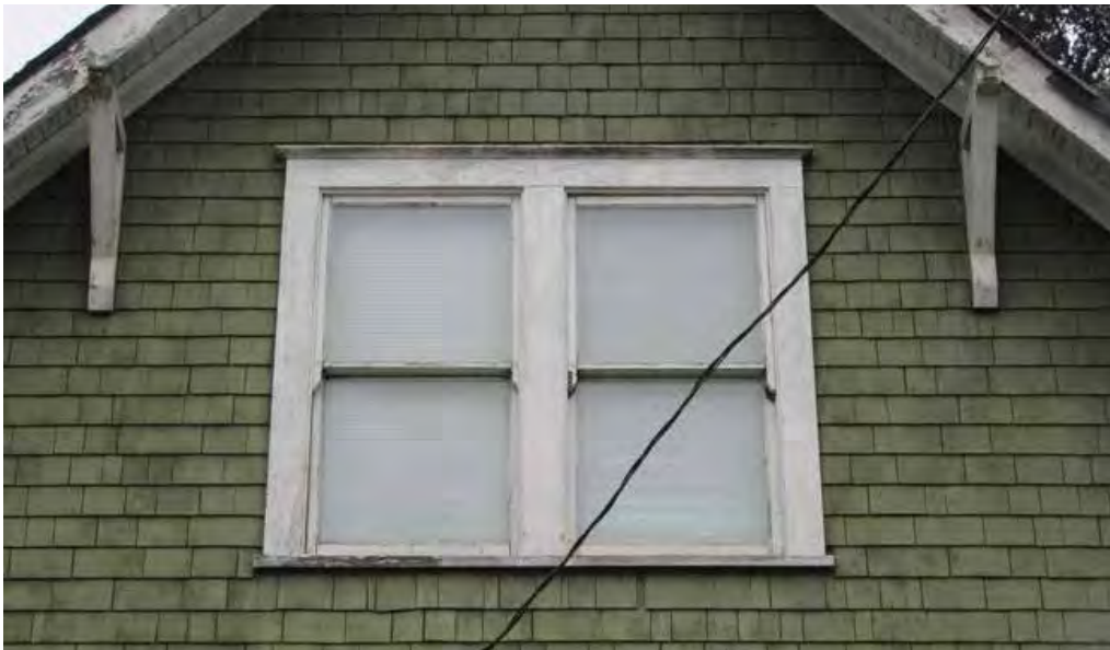
Pair of original one-over-one, double hung wooden sash windows on second storey of front façade
