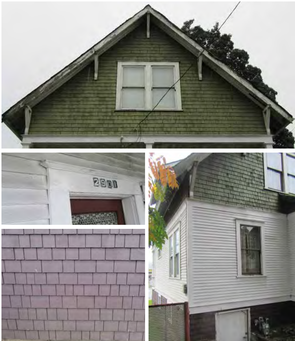
Clockwise from Top: Shingle siding at second floor; Lap siding, belt course, watertable and cornerboard; Shingle siding at basement; Door trim
