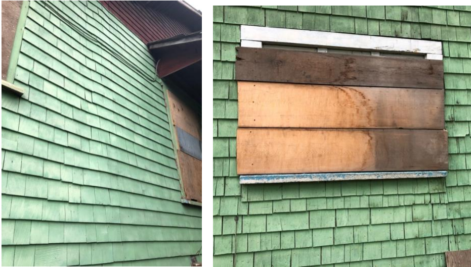
Figure 12: Example of Irregular Application of Cedar Shakes – north side (left), south side (right). The former illustrates the joining of the later addition to the original house while the latter illustrates either an enlargement or alteration to the original window and the siting of the sill.
